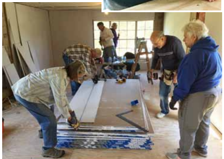
Paula Schaffner, Dick Horstman, Ron Guidry, and Judy Horstman work together on hanging sheetrock, while in the background, John and Mary Moritz work on electrical and clean windows.
