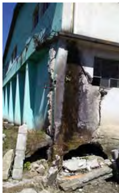
Religious Education Building in dire need of stabilization.
